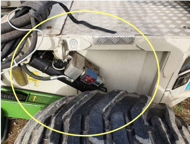
Fig. 3. Moog valve block with an ICM. The new actuators are mounted on the HFE joints to enable accurate and responsive chassis balancing.
