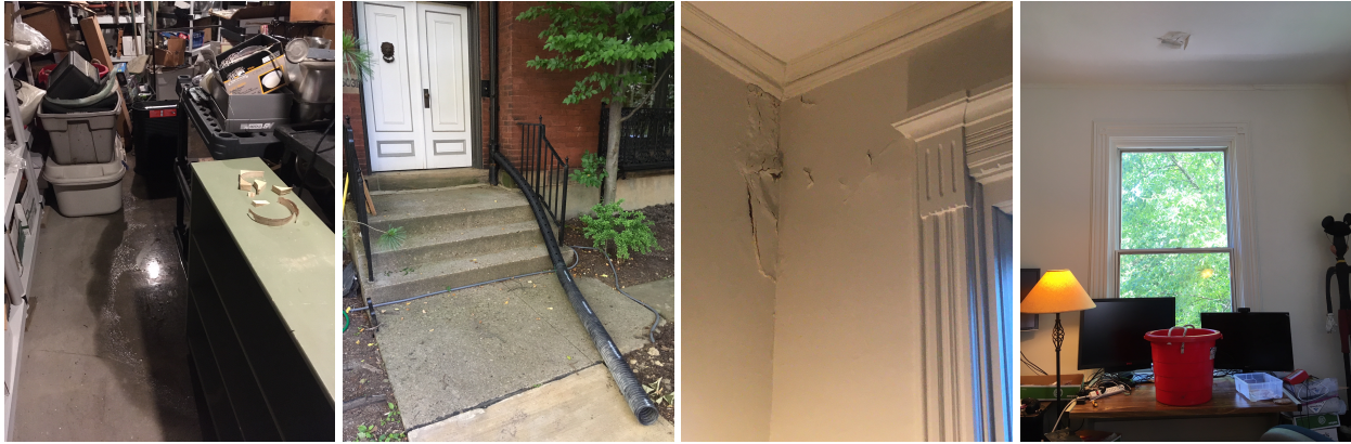
Figure 3: The learning challenges of owning an old home. Left to right: the waters 2 days after a basement flood, the downspout bypass, the bubbling plaster in the dining room, and the leak in my home office,
