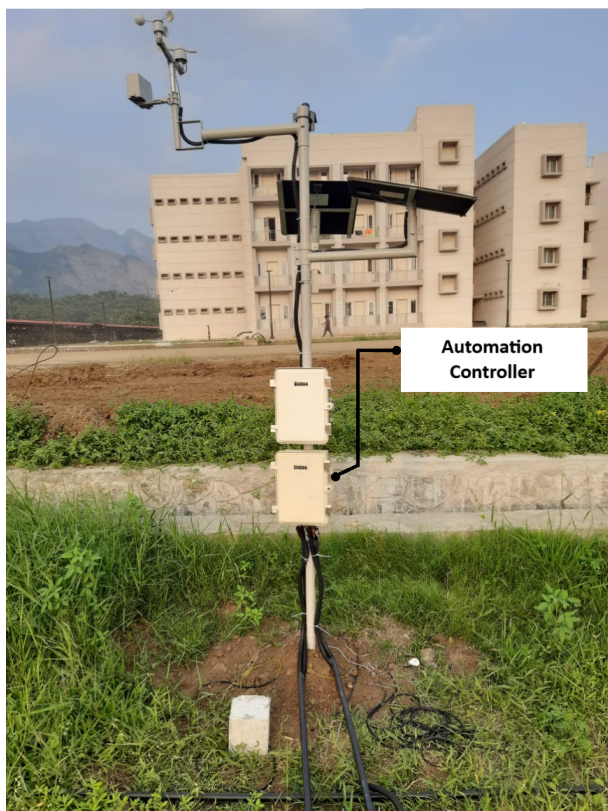
Figure 4: Automatic Drip irrigation controller installed on a pole with Weather station System.
