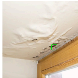
a roof leak forming on a ceiling .
