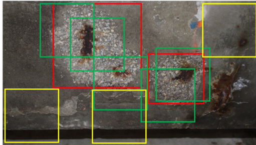
Figure 3: Extracted patches from spalling dataset image. ‘Red’ - labelled spalling region, ‘Green’ - spalling extracted patches, ‘yellow’ - non-spalling extracted patches.
